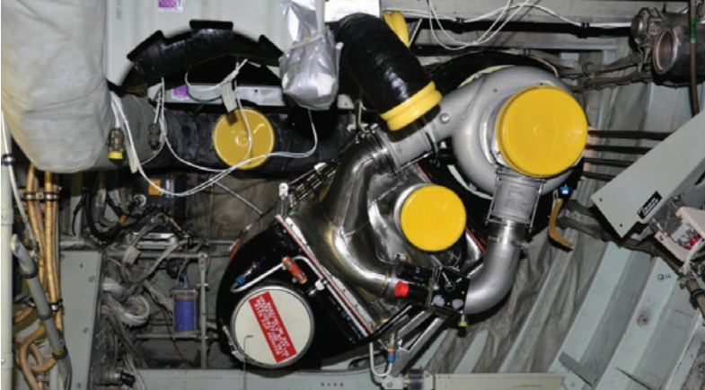
New ECS Refrigeration Unit
